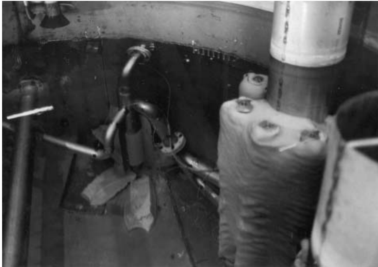
Figure F(a). Ringhals 1 strainer system some time after cleaning of the wing strainer when a further build up of debris on the wing strainer has occurred
