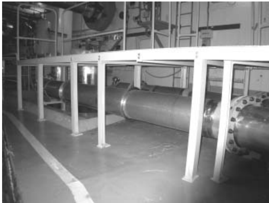
Figure O. The horizontal sacrificial strainers at Ringhals 2
