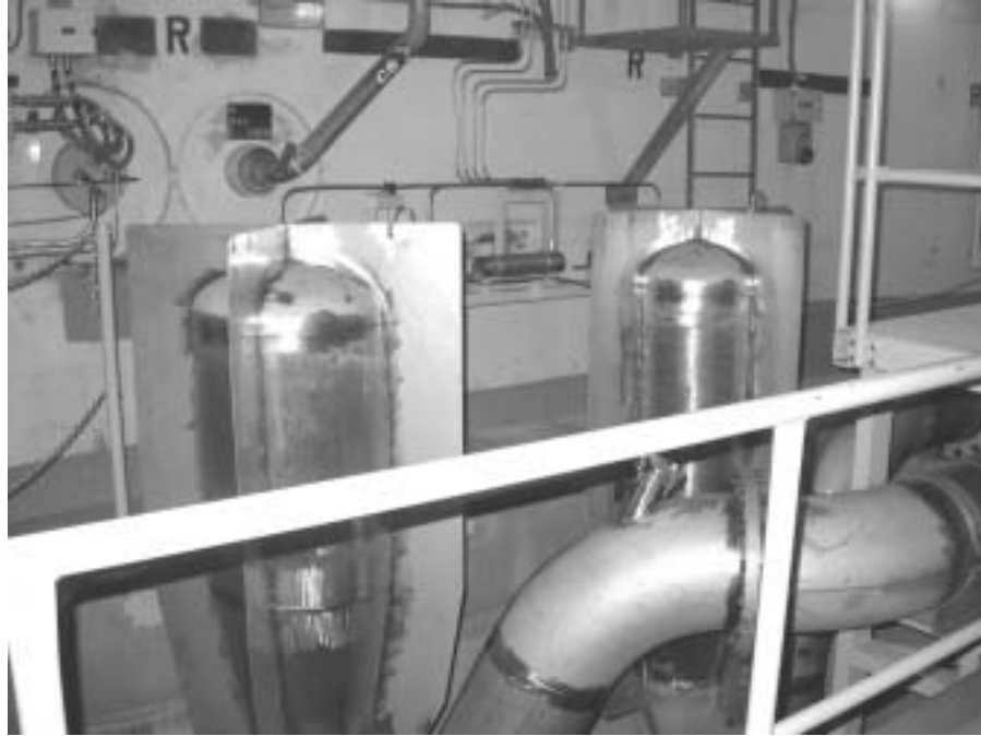
Figure N. Self-cleaning wing strainer at Ringhals 2 NPP
