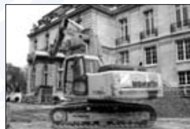
Work begins on the renovation of the La Murette site and the construction of a new conference centre.
