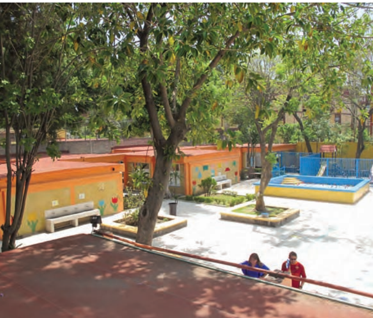
Figure 3.4 ■ Roof waterproofing membrane, Escuela Mexico Olimpico, Jardin Balbuena, Venustiano Carranza, Mexico D.F © Alastair Blyth
